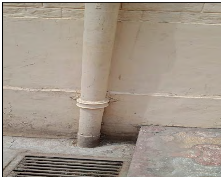
Fig.3.2: Rain Water Harvesting System on the college campus
